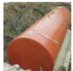
Underground Storage Tanks
