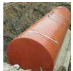
Underground Storage Tanks
